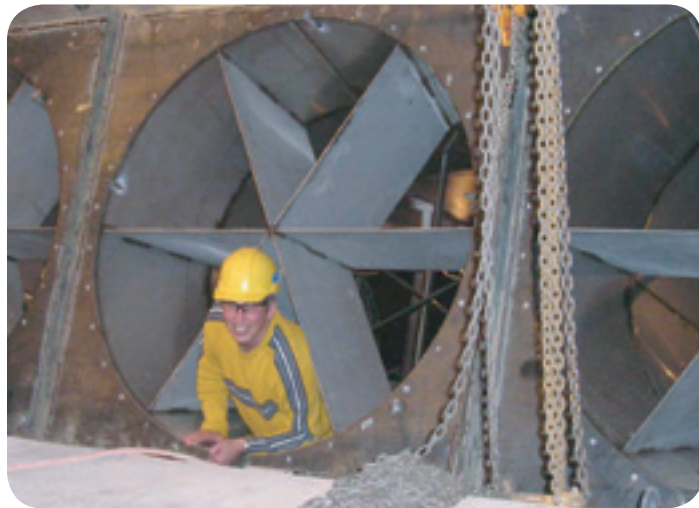
Installation of multiple High Beta® Elements within a rectangular duct, focusing on the straightening vanes
